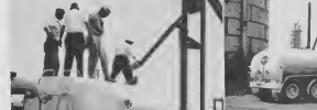
THE FIRST delivery of penetration asphalt for the Princess Beatrix Airport construction project was made Sept. 9. A 9000-barrel tank and special swivel delivery arrangement were constructed south of the Central Tool Room. E. HUYBREGER entrega di azific na serventor Frances Broux, caminda un proyecto di construcion ta sumando haba, a wordo hiba 9 di September. Un tanki di 9000 barrel cu su tubo especial ta equipo cu un wordo traha.
